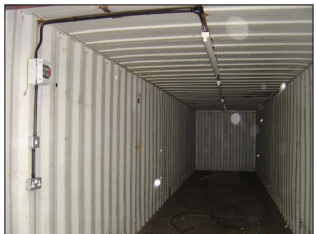
40' Standard - Electrics & Lighting
